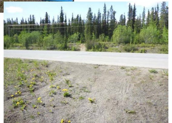
Highways and major roads bisecting the network; uncontrolled and unsafe crossings
